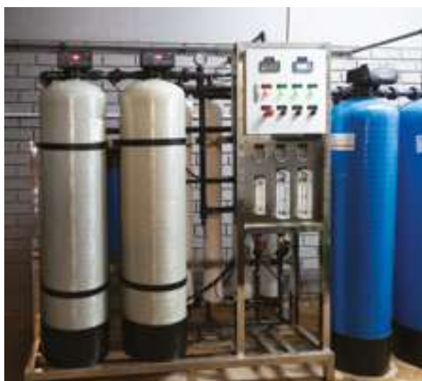
Water purification system
