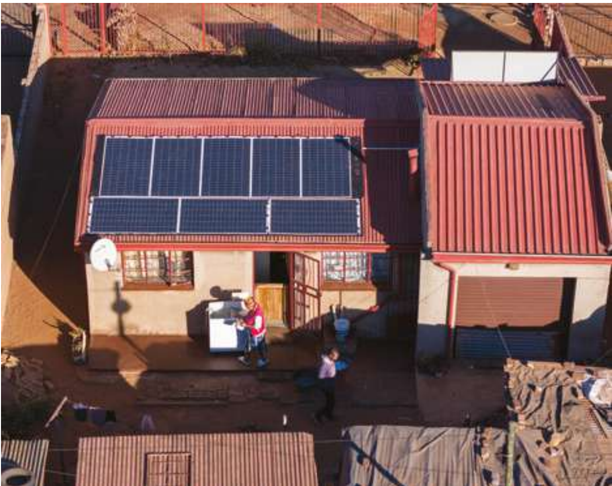
Installed Wetility solar
